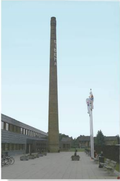
This chimney is subjected to the combined loading of wind and weight. It is important to investigate the tensile stress in the chimney since masonry is weak in tension.
