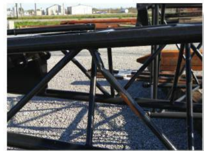
Failure of this crane boom was caused by the localized buckling of one of its tubular struts.
