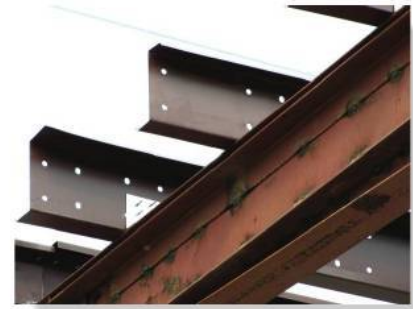
Zee sectioned members are often in light-gauge metal building construction to support roofs. To design them to support bending loads, it is necessary to determine their principal axes of inertia.
