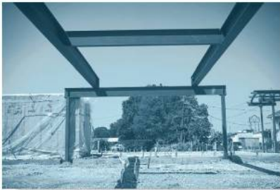
In order to design the horizontal members of this building frame, it is first necessary to find the internal loadings at various points along their length.
