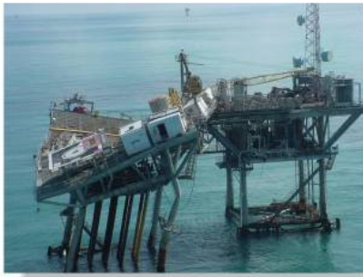
The dramatic failure of this off-shore oil platform was caused by the horizontal forces of hurricane winds, which led to buckling of its supporting columns.
