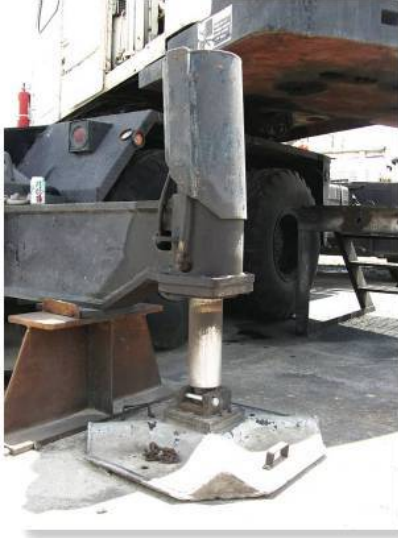
Cranes are often supported using bearing pads to give them stability. Care must be taken not to crush the supporting surface, due to the large bearing stress developed between the pad and the surface.
