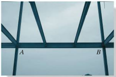
The two floor beams are connected to the beam AB , which transmits the load to the columns of this building frame. For design, all the connections can be considered to act as pins.
