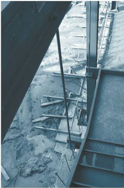
This steel tie rod is used as a hanger to suspend a portion of a staircase, and as a result it is subjected to tensile stress.
