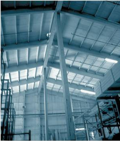
These long unbraced timber columns are used to support the roof of this building.
