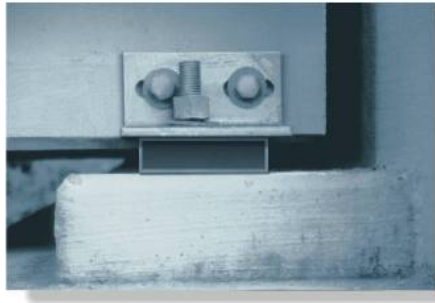
The rubber bearing support under this concrete bridge girder is subjected to both normal and shear strain. The normal strain is caused by the weight and bridge loads on the girder, and the shear strain is caused by the horizontal movement of the girder due to temperature changes.
